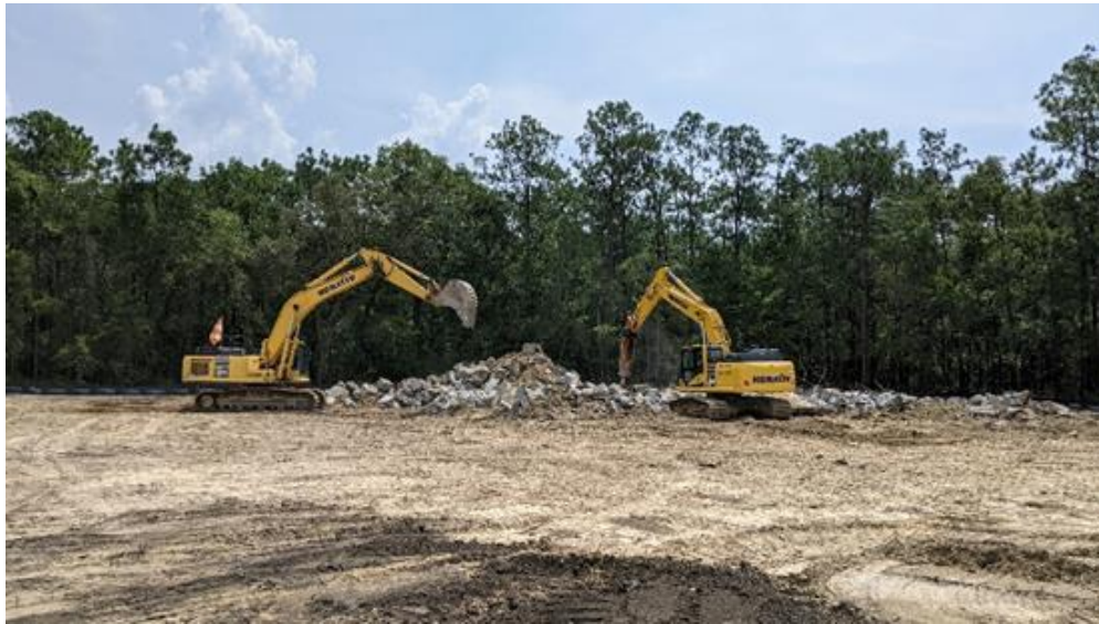
Photo 1.8: Piled demolished concrete being turned into crushed concrete via vibratory hammer excavator attachment.
