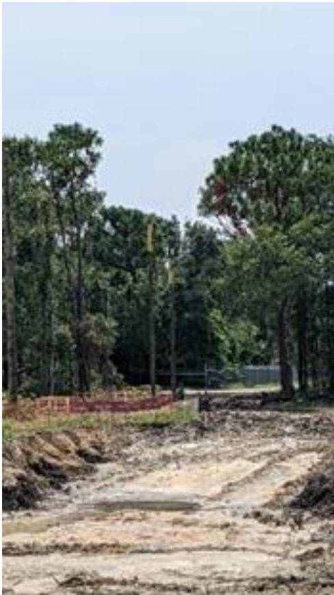
Photo 1.12: Newly installed Gulf Power/NextEra Power poles for routing of new line around exterior of the project with demolition of the existing line to follow.
