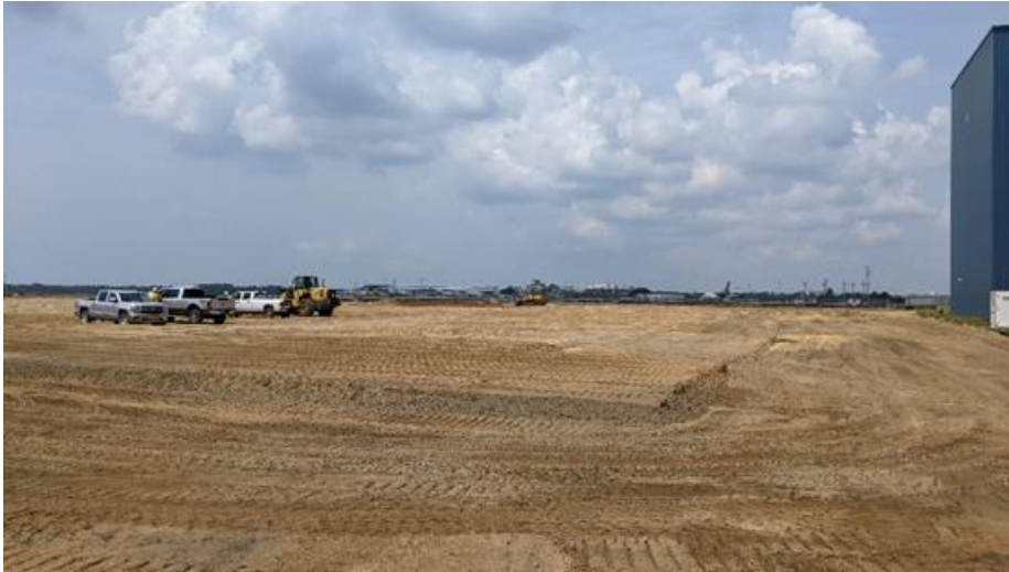
Photo 1.11: Compacted lifts for Hangar 2 pad. Also shown on the right is the demolished existing drive/walkway.
