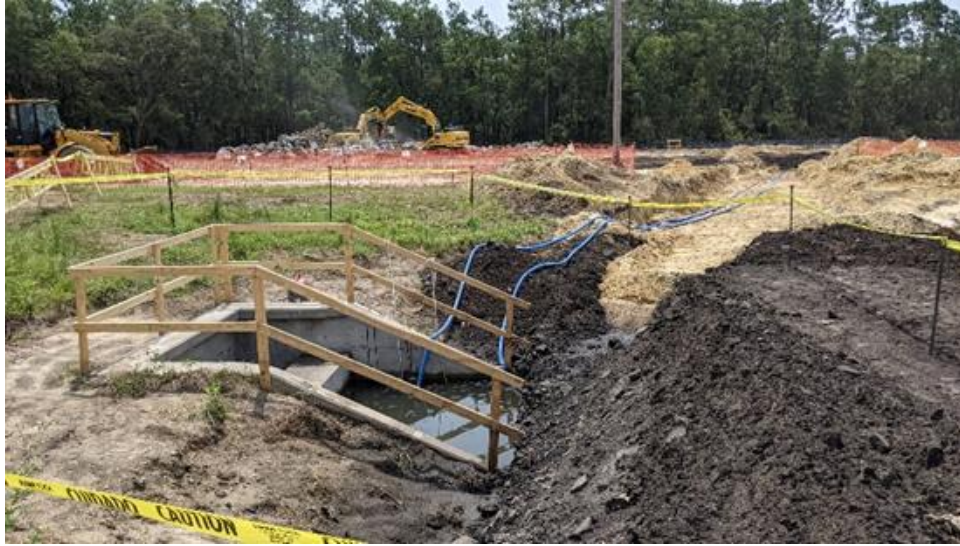
Photo 1.7: Safety procedures around separated dewatering area with appropriate caution tape and guardrails.
