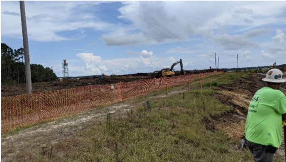
Photo 1.2: Earthwork Subcontractor clearing and grubbing. Labeled and delineated power line crossing area.
