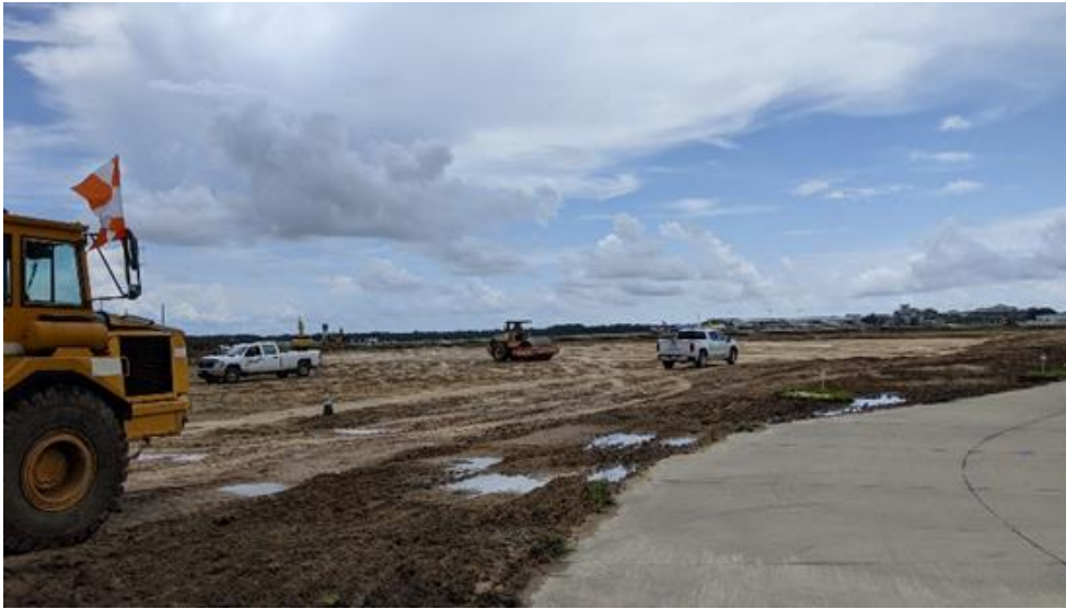
Photo 1.1: Earthwork Subcontractor continuing to cut and compact new hangar pad to appropriate elevations.
