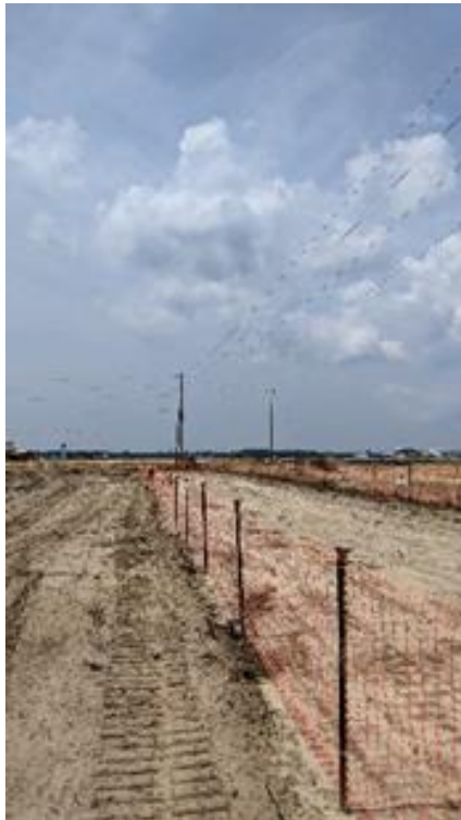
Photo 1.10: View of barrier in relation to overhead power lines.
