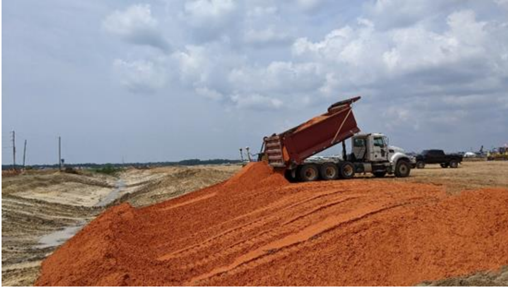
Photo 1.5: Suitable material being brought in to bridge the water in existing drainage ditch.
